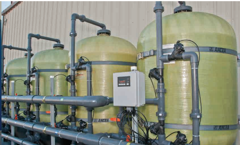
Parallel 48" x 72" Quad Carbon filter system with sequential backwash.
